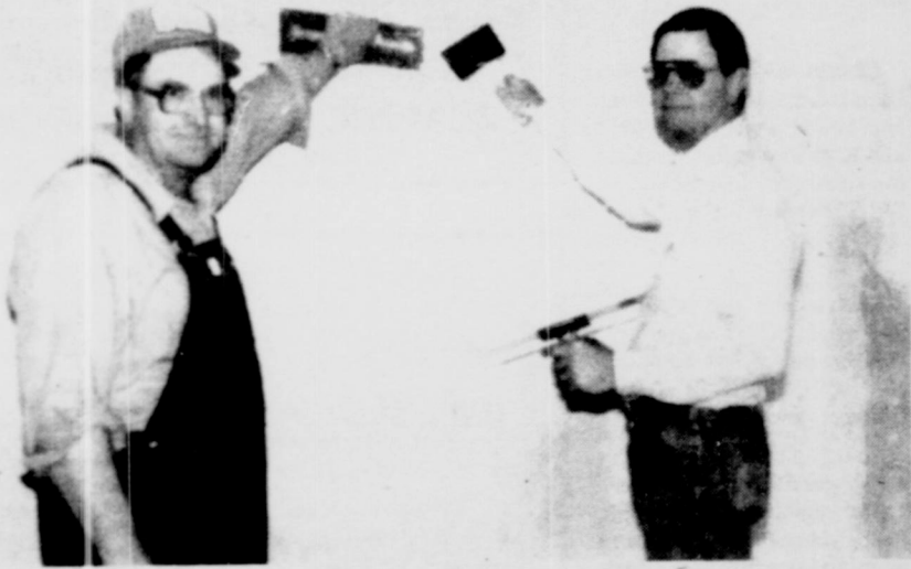
Greg Lamb and Bill Homer put the finishing touch to the walls at the Community Center preparing for them to be painted.
