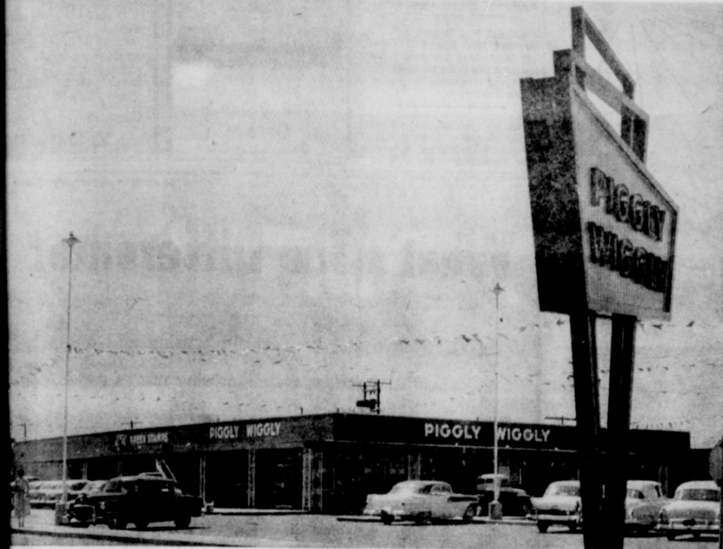
PIGGLY WIGGLY'S NEW BUILDING located between Lubbock street and Panhandle avenue is now under construction.
