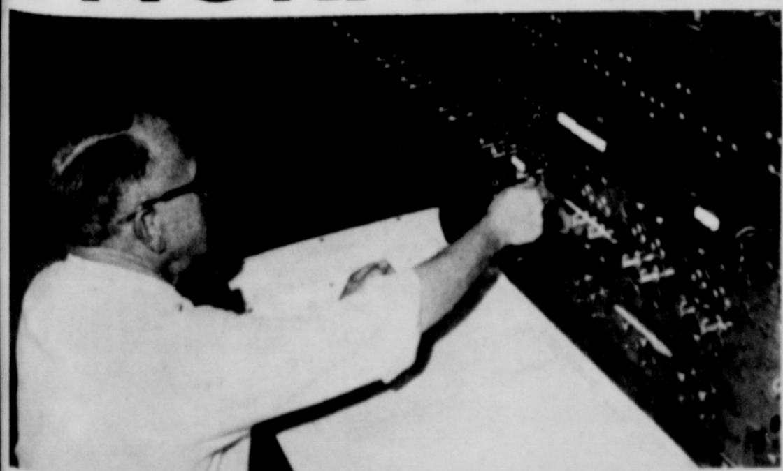
CONTROL BOARD--Bill Roche, dispatcher for Santa Fe, is shown at the traffic control system board--a system that controls trains over much of the Slaton Division.
