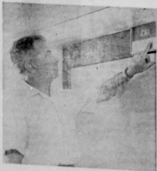
Mr. Sims points out the simple control on the electric air purifier which automatically rejects pollen, dust and other irritants, giving the Sims family clean, fresh air throughout the home.
