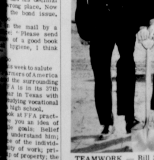
TEAMWORK — Bill Smith and son Steve teamed up on the shovel to break ground for the new Smith Ford, Inc. building here last week. The huge new automotive plant will be located on the US-84 bypass at the west end of Division Street. (SLATONITE PHOTO)
