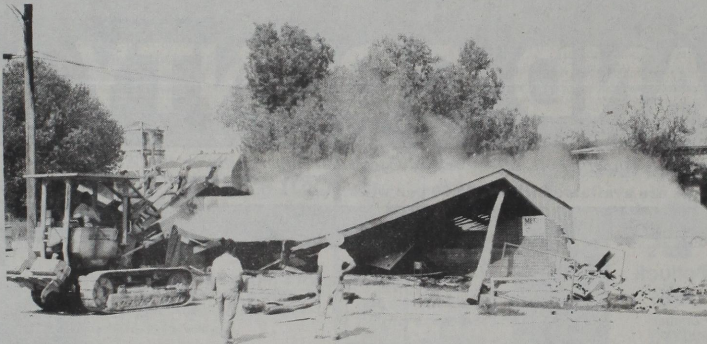
The dust rose as the wall hit the ground and the last obvious vestige of a grocery store that served the community for many years became rubble to be pushed into the former basement and covered with dirt Friday afternoon.
