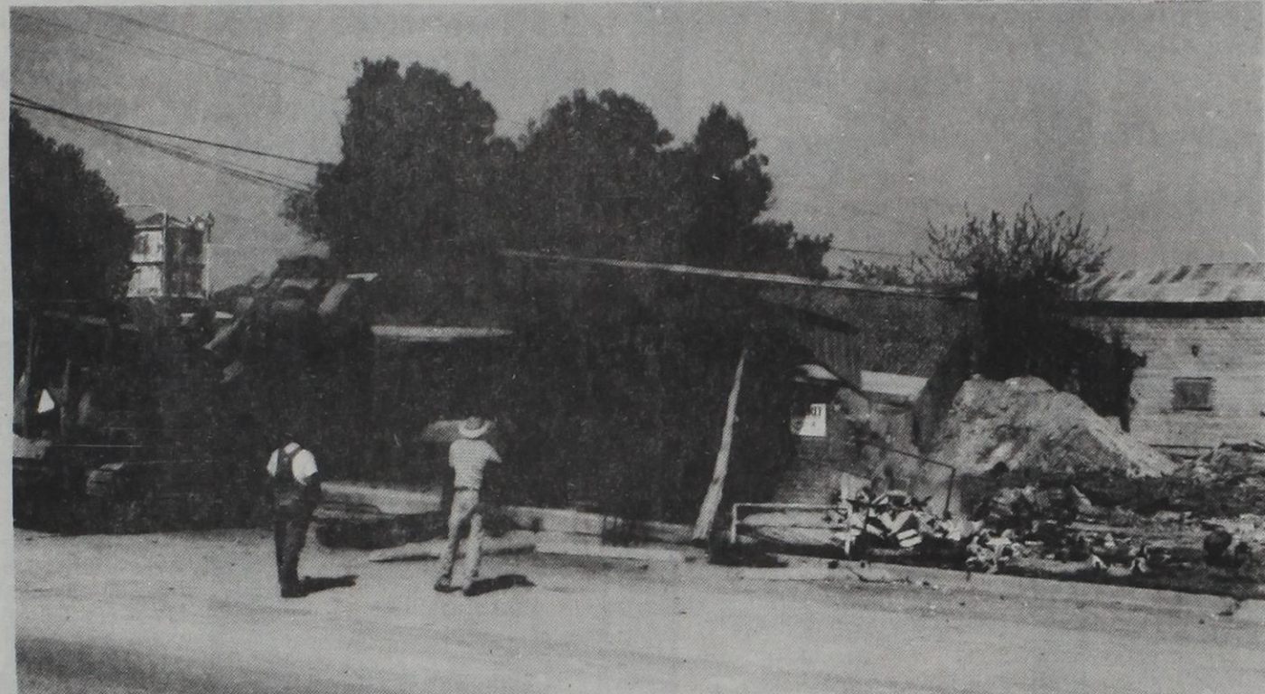
The front wall of the former grocery store was given a shove by equipment operator Don Cornett as Bostick and Bush looked on Friday afternoon.
