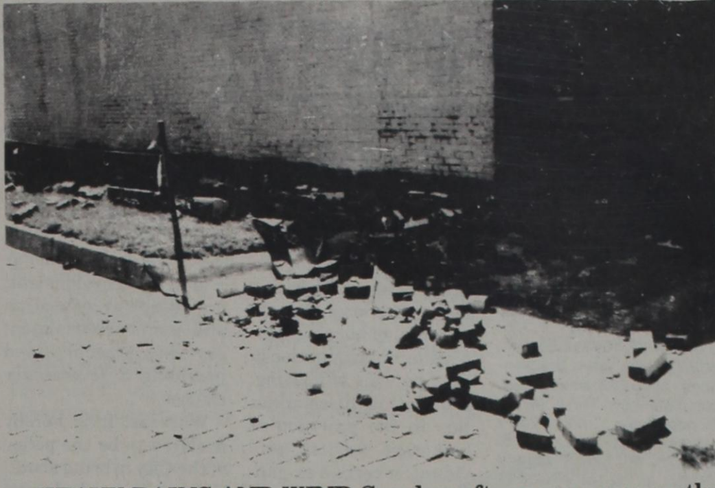
HEAVY RAINS AND WIND Sunday afternoon apparently caused brick to fall from the building located at Conrad Hilton Avenue and East 5th Street. The building formerly housed Darr's Automotive Shop, and is owned by Vera Darr. (Staff Photo)
