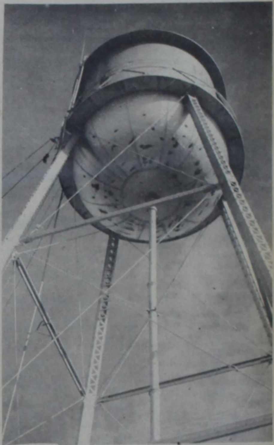
WELDING SCARS - - Black patches of blistered paint from the heat of the interior welding show on the bowl of the water tower. These were sanded and repainted.
