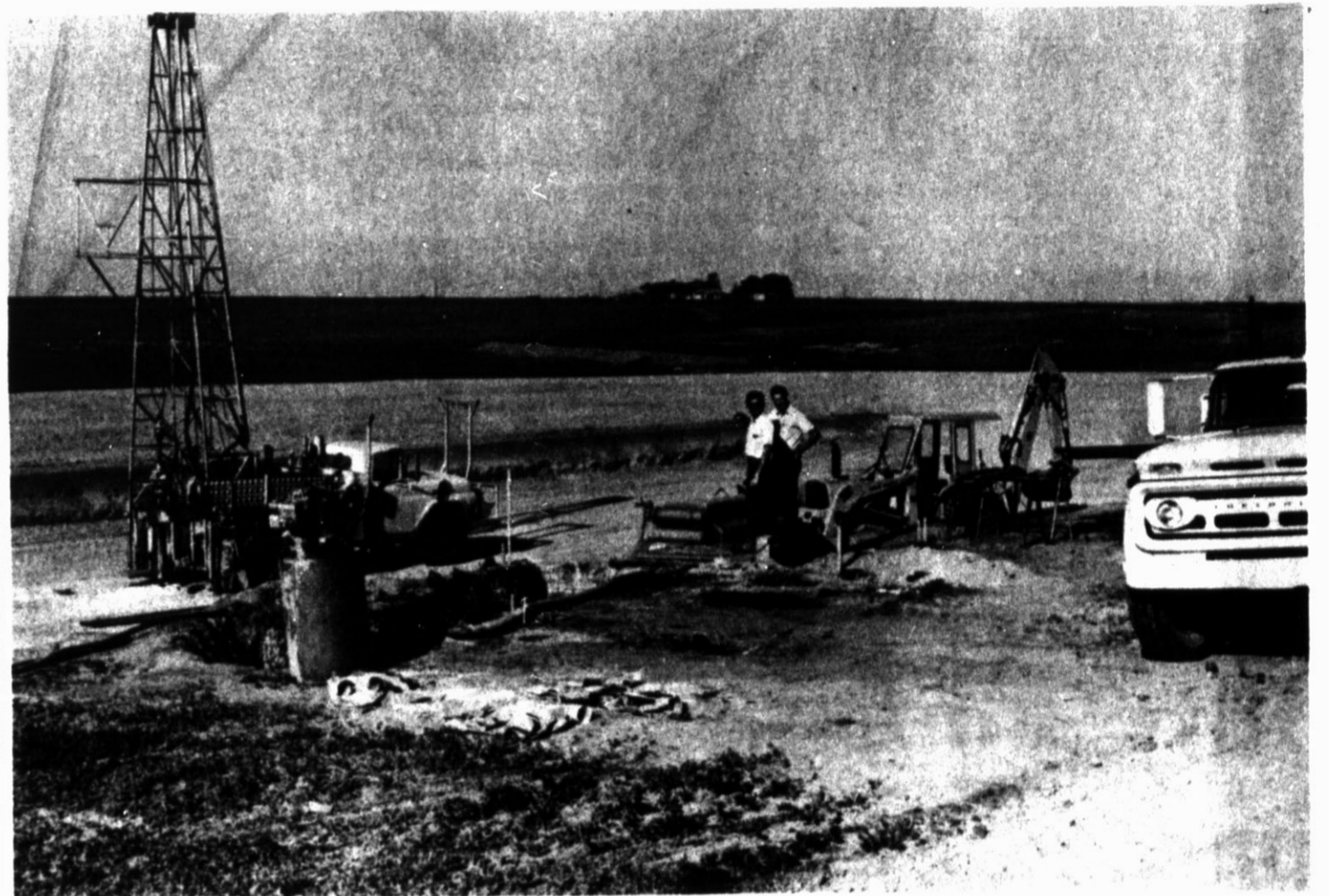
RECHARGE SYSTEM — J. C. Brown, right, with the Soil Conservation Service, and Arland Schneider, research engineer, look over the first water recharge system ever constructed to restore water
