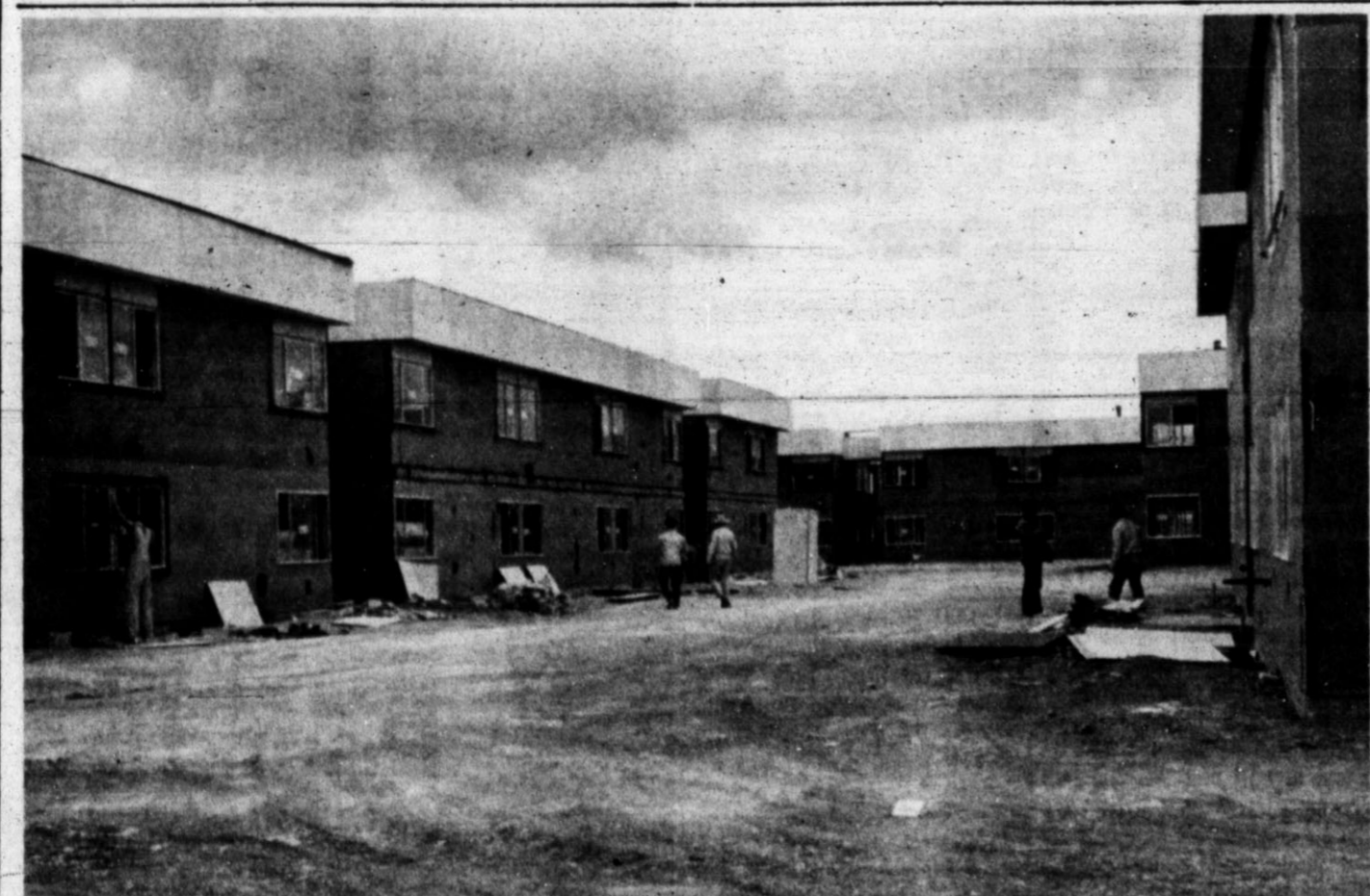
WORK CONTINUES — Construction work on the Blue Water Gardens Apartment complex in northeast Hereford continues with an early July deadline set for the opening date of three of the 12
