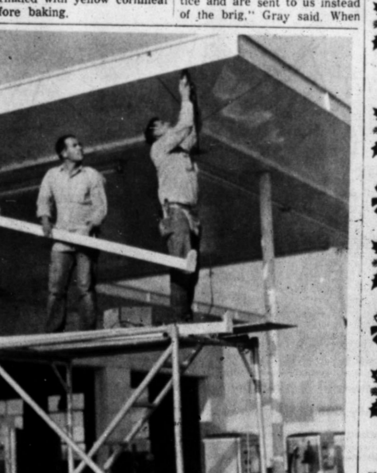
SIGNS OF PROGRESS — These workmen were found Monday afternoon doing repair work on the roofing of a service station on E. Highway 60. There is a lot of this type work being done lately as Hereford prepares for the winter. (Hereford Brand Photo)
