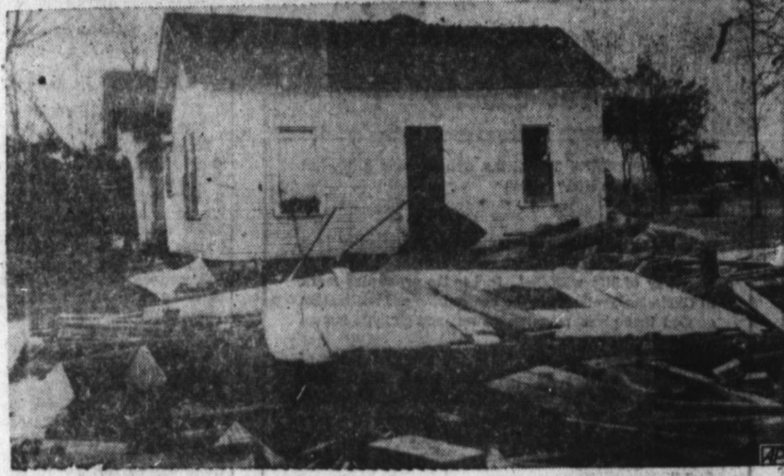
TWISTER LIFTS HOUSE —The home of Mrs. Porter Rushing of Port Neches was lifted 15 feet off its foundation by a twister that rip-
