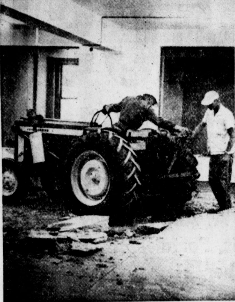
TRACTOR IN THE BASEMENT of the county courthouse is really tearing things up. With all of the partitions down, the tractor is ripping out the concrete floor, which will be replaced with terrazzo. The activity is part of an extensive renovation of the 50-year-old building. (Staff Photo)
