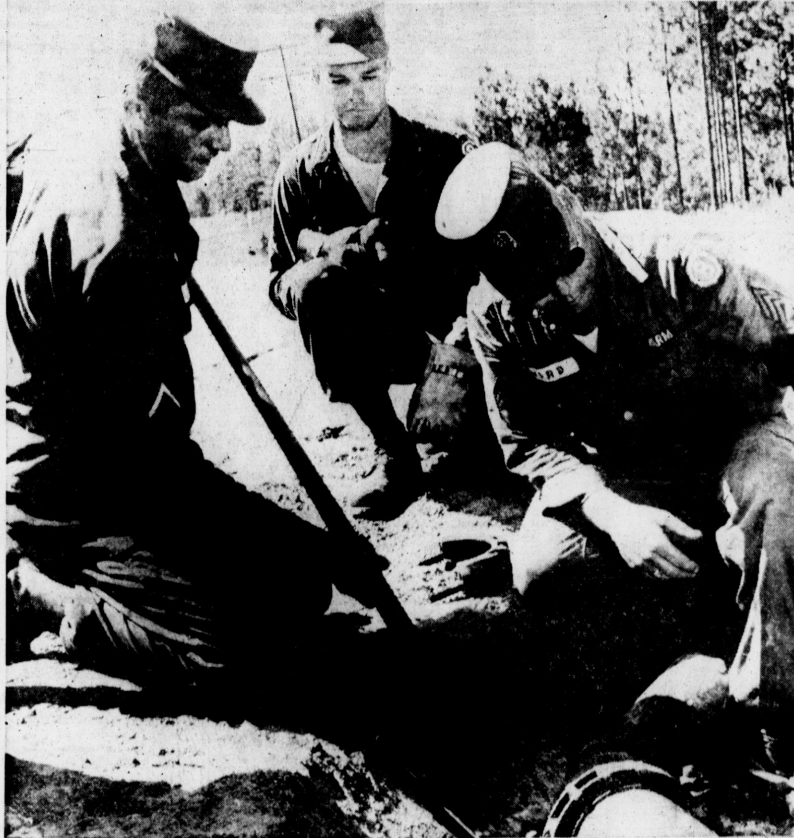
PIPELINE PROJECT—Shown are PFC Richard J. Zinser and PFC Wallace S. Woolsey, pipeline builders, at left, both of Hereford, and Sgt. Willie J. Word, pipeline supervisor, of Dimmitt, as they lay pipe at annual active duty training for army reservists at Ft. Polk. These men are members of the 700th Engr. Co. (Pipeline), attached
