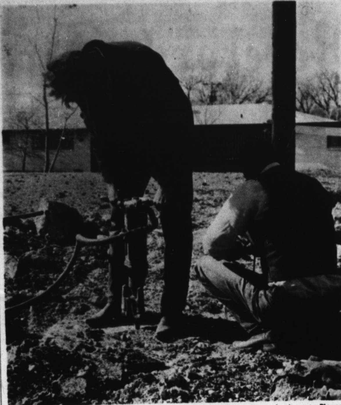
DRILLS ROCKS —Workmen drill through rock near the creek bed to clear a way for a ditcher to lay the new four-inch line to replace a smaller pipe to feed gas to Pioneer Natural Gas Co. lines. See story page 1 (Staff Photo)
