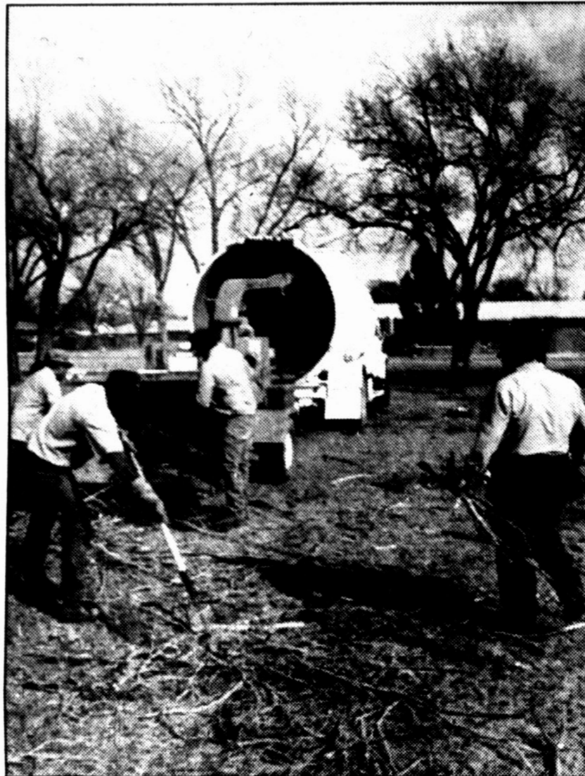
Work at the lodge — City workers shredded trees, branches and twigs at the old Campfire lodge. Some of the ongoing work follows in the wake of an ongoing controversy regarding the use of the facility.
