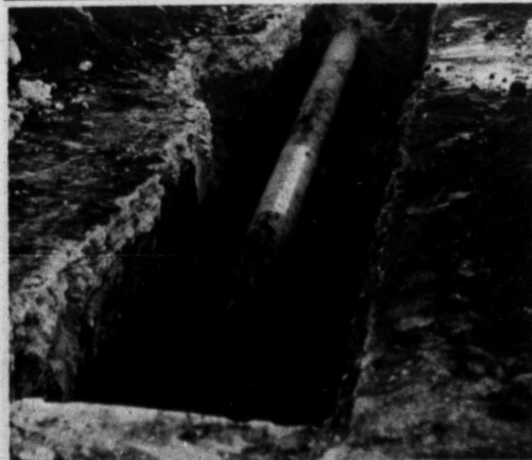
ALL FIXED! Pioneer Natural Gas repaired a leak on one of its main lines on the corner of 6th and Main. The leak was discovered during the last survey which the company makes four times a year. (Hereford Brand Photo)
