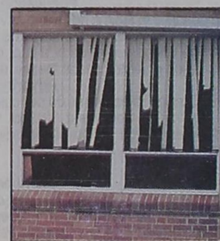
Like skeletons in the wind, vertical blinds, shredded by large hail, flutter behind broken windows of the Gruver High School Administrative office.
