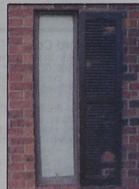
Large hail made good-sized holes in the shutters on the home of Margaret Ralston on Cooper Avenue in Gruver.
