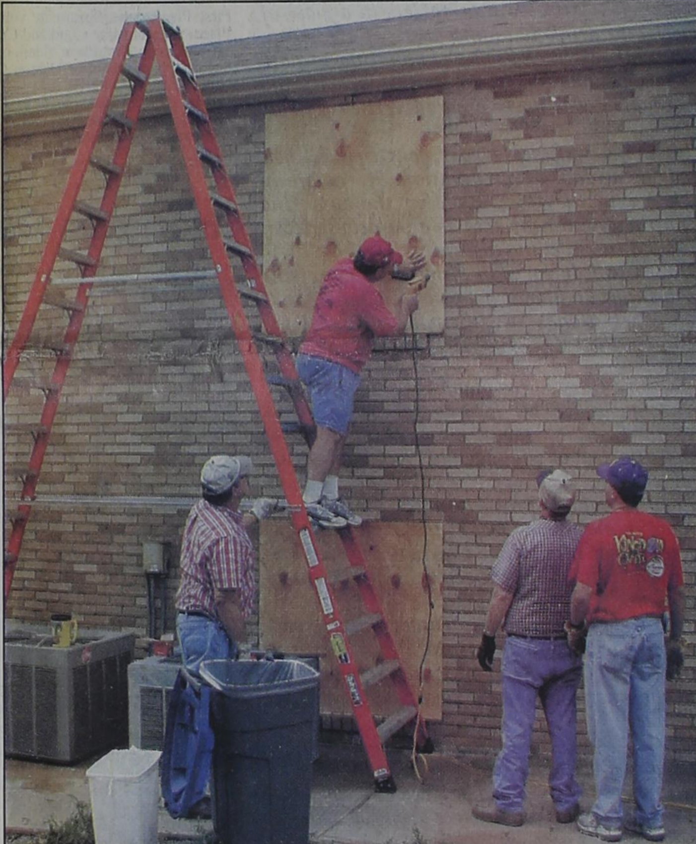
Mack Hoel nails plywood over the north windows of the First Baptist Church. Helpers Kermit McKee, Bill Heddins, and Scott Curry assist in the work.
