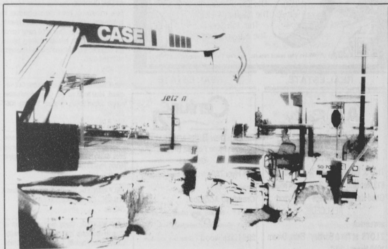
OUT WITH THE OLD - The Spearman Allsup's gas tanks are getting a face lift. A crew from out of town came in to replace the old leaky tank. Construction is not expected to last long. (photo by Chad Davis)
