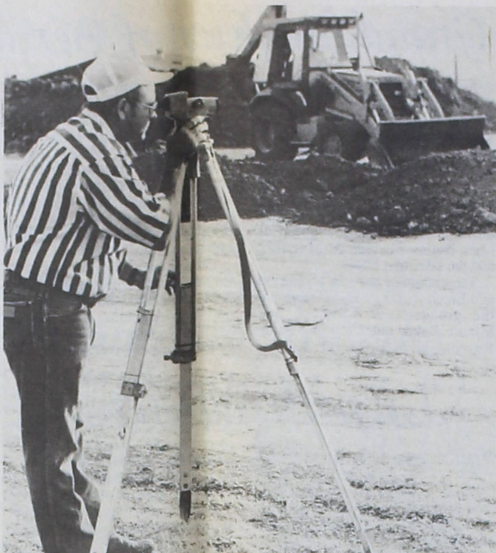
PATRICK H. WHITE of Valley View, an independent contractor, surveys the future site of Muenster ISD's new gymnasium. White was hired by the school district to supervise construction which began last week. Bernard Hesse of G&H Backhoe Service is seen working in the background.
