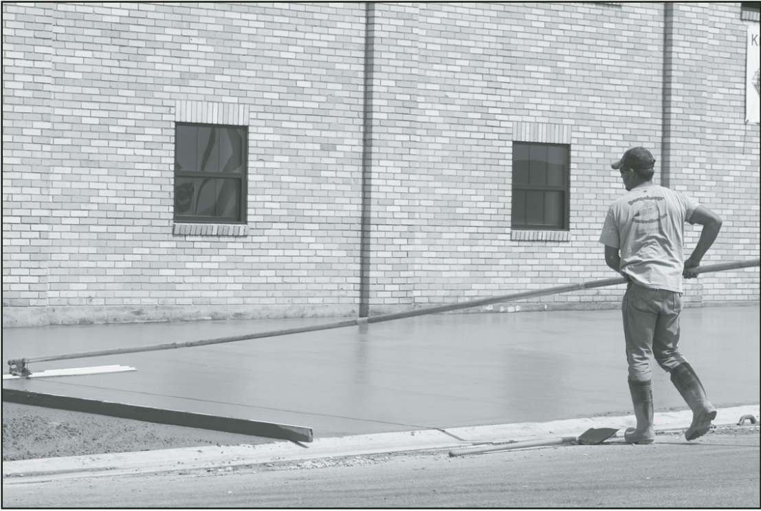
Progress continues high and low at the Muenster Knights of Columbus Hall, including the placement of new windows, and new paving around the building. Janie Hartman photos
