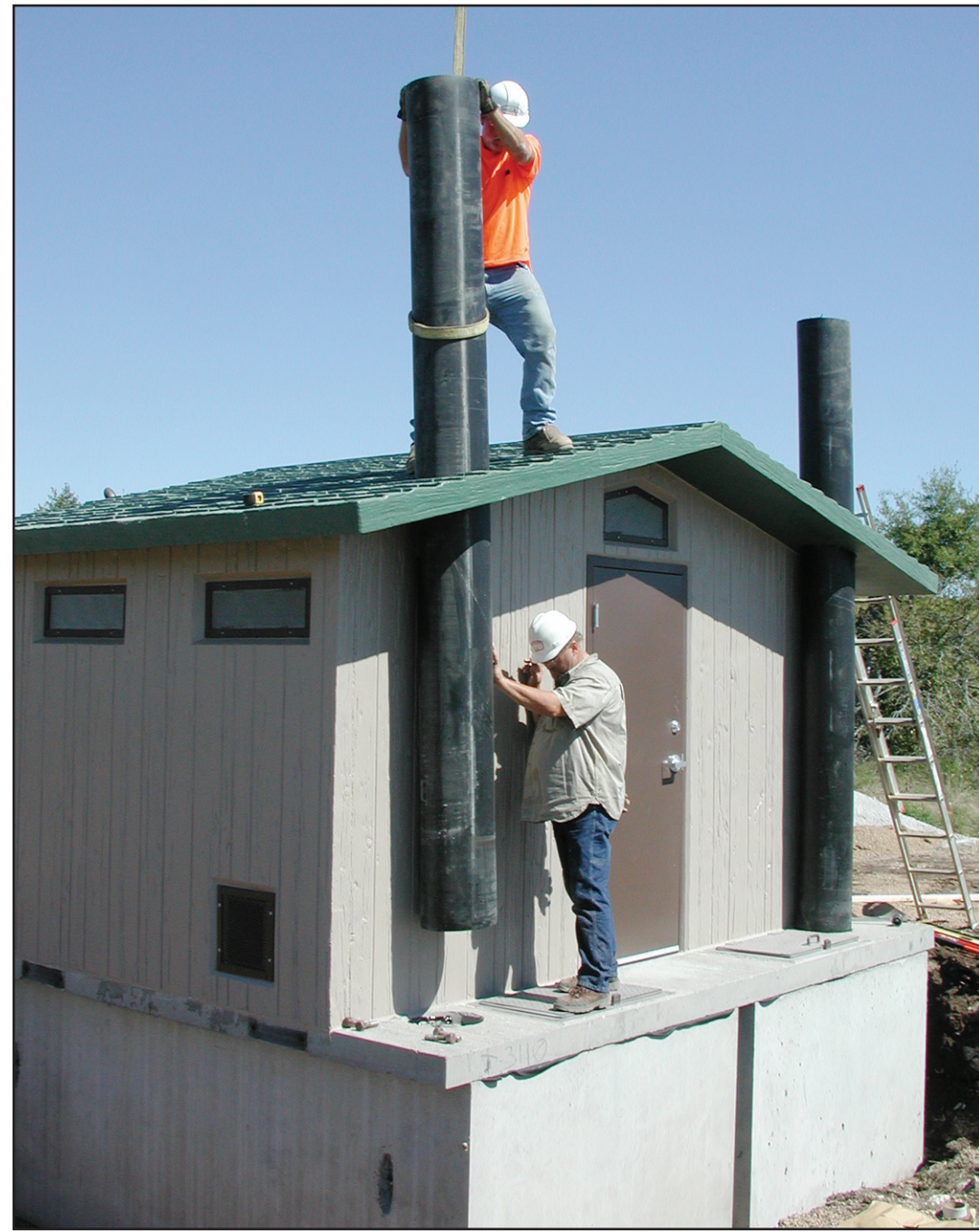
Crews installed the new restrooms just north of the parking lot near the boat ramp at the west lake access area last week. Called a Tioga Special, the concrete building and vaults weigh 73,200 pounds. Black vent pipes (pictured being installed) are located on the back side (south) of the building in order to be heated by the sun, to create a positive continual air flow from the vaults. The cost of the restroom was $24,228 and will be paid 75% by the TPWD Boating Access Grant and 25% by Muenster Water District funds. Courtesy photo
