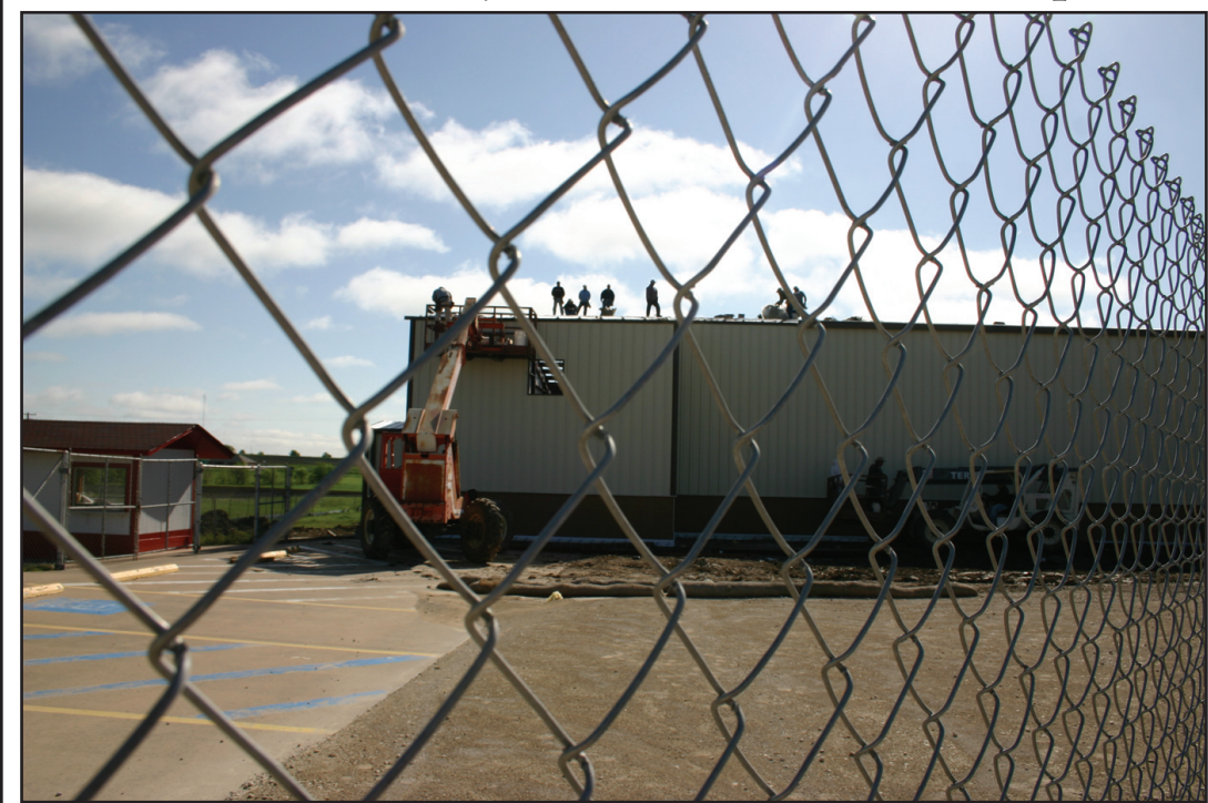
Work continues inside the fenced off area of the used-to-be Hornet Stadium parking lot, as the outside walls of the new practice gym building near completion. Janie Hartman photo
