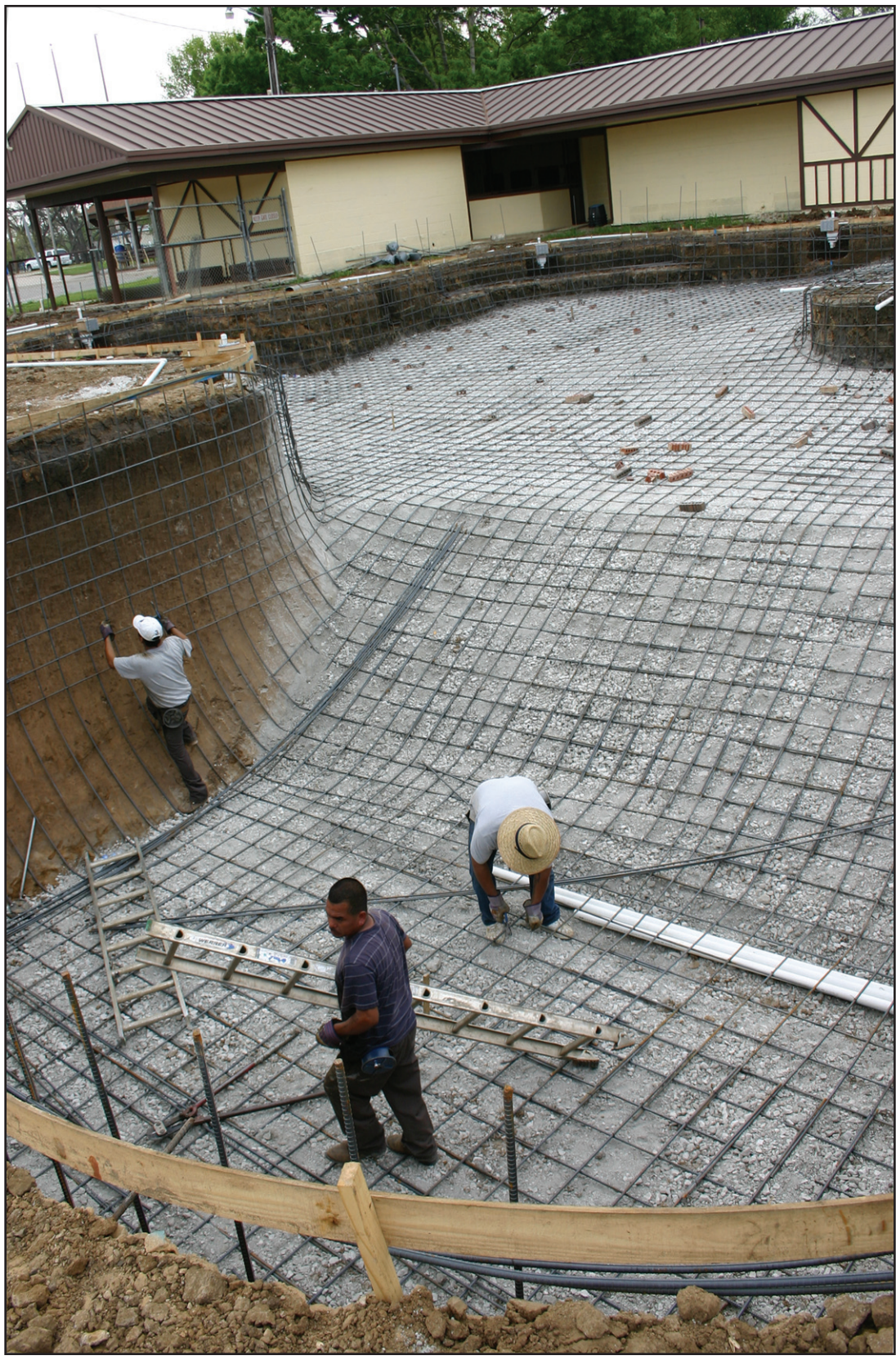
After experiencing a late start due to rain and mud, work is in full swing on the new Muenster swimming pool in the City Park. Its exciting new shape will allow several requested features including a lap area and spray feature. Janie Hartman photo
