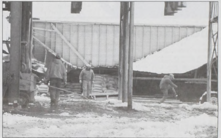
Too much snow causes a roof to collapse at Tony's Seed and Feed. Scott Wood photo
