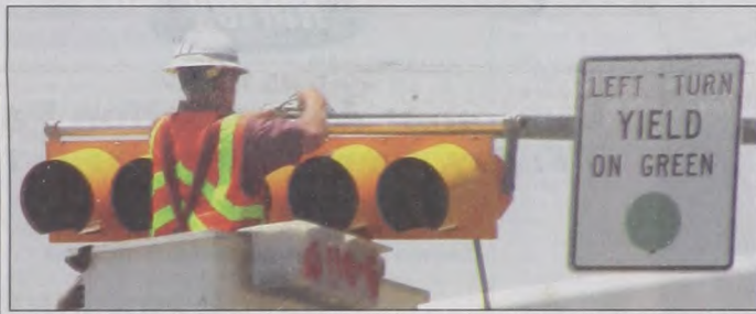
Texas Department of Transportation installed new lights at the U.S. Hwy. 82 - FM 373 intersection Tuesday afternoon. The 5-head signals will allow vehicles to turn left off of Hwy. 82 during a green arrow or solid green light. Janie Hartman photo
