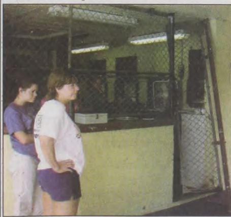
Muenster Swimming Pool Manager Shirley Hess, right, and lifeguard Kim Hess observe damages done late last Wednesday night or early Thursday morning when illegal access was made to the facility. A chained gate was yanked loose to gain access to the office area. Damage occurred to locked cabinets that were pried open and ransacked. The only cash kept there was lifeguard tips estimated at between $50 and $60. During that same time frame Doc's was also broken into. Muenster Police Chief Bob Stovall said that at 3 a.m., he discovered the rear glass door had been broken into. A search of the facility found nobody there. Only a bottle of whiskey was listed as missing. Chief Stovall said that he feels both burglaries had the same people involved. He also has an idea that some of the recent burglaries are alcohol related. Anyone with information is asked to contact him at 759-2236.
