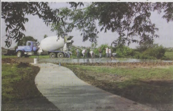
Concrete pours from a Walterscheid Construction and Redi-Mix truck on Wednesday morning as workers from Dangelmayr Construction, Inc. smooth out the wet mix. They are working on the helipad for medical helicopters to land. It is located south of Muenster Memorial Hospital. A sidewalk was also built to the site from the Hospital.
