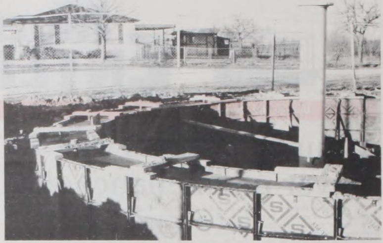
Concrete footing is poured at the site of the new water tower.
