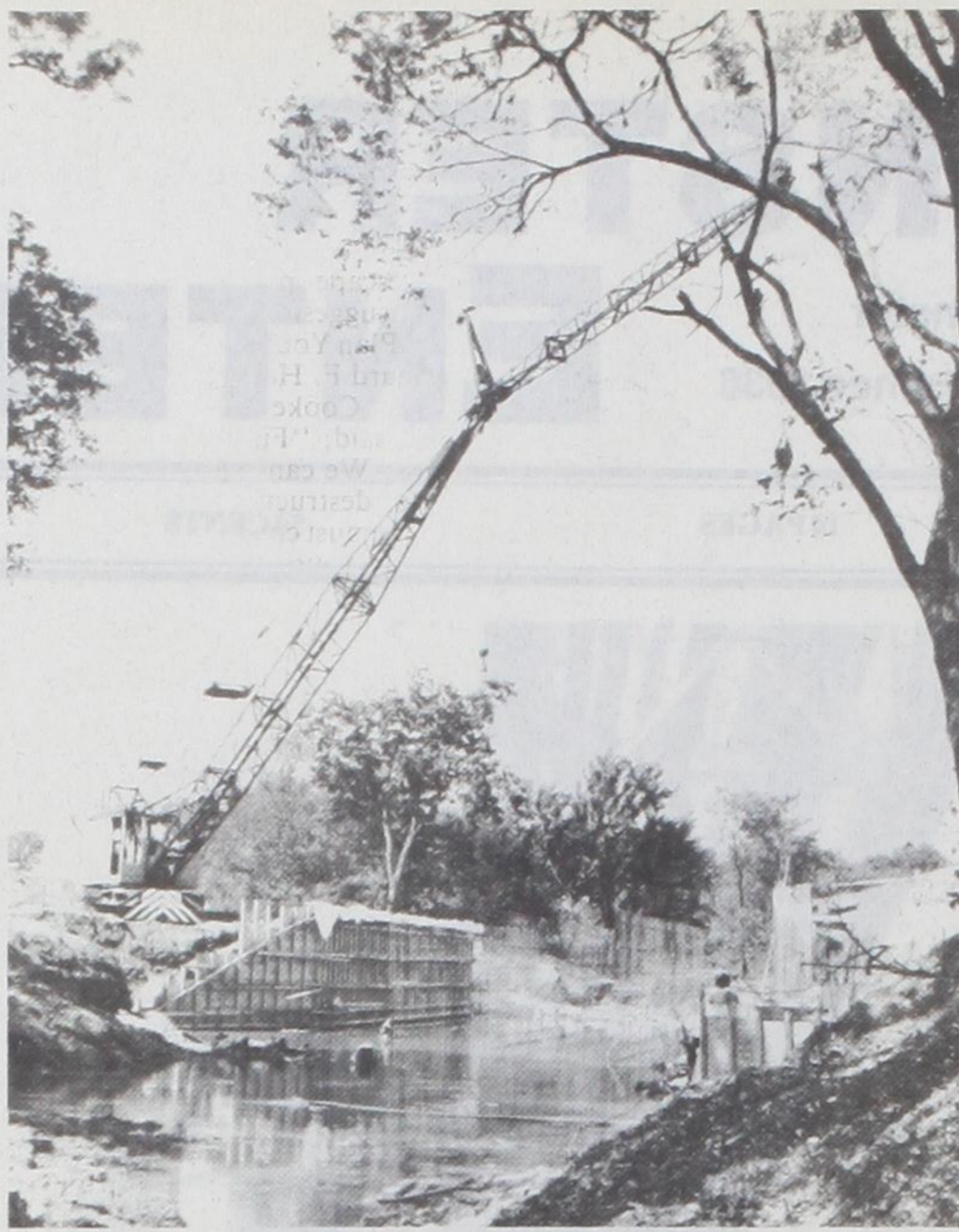
A NEWLY CONSTRUCTED BRIDGE will soon span Brushy Elm Creek on Copper Switch Road, about 4½ miles northwest of Muenster. The bridge is being replaced as part of a federal bridge program with the federal and state government paying the majority of the bill and the remainder already paid for out of Precinct 4's last budget. There was a problem with the last end gravel washing out during heavy rains where the creek curved at the bridge. To remedy this, the creek channel has been changed and a four-barrel box culvert-type bridge is being installed. Sub-contractors Schuster and Walker are installing the bridge for the actual contractor, Rushing Paving Co. Janie Hartman Photo
