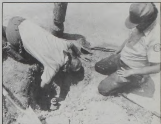
CHRIS YOSTEN (right) and David Dittfurth fix a troublesome water leak under Main Street at the corner of First and Main. City employees will soon have much more time for street, water and sewer maintenance when Texas Waste Management, Inc. takes over the garbage collection job. Janie Hartman photo
