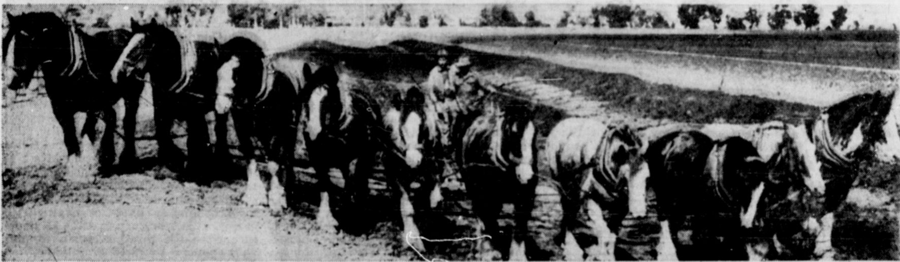
TEN HORSEPOWER DIGGER IN ACTION —In these days of power-driven machinery, a ten-horse team is a rare sight even in Australia. This ten-horse team is in use in building an irrigation canal in the Murray Valley soldier settlement near Victoria, Australia, where between 500 and 600 miles of irrigation channels are being excavated. Horses are being used in moving the dirt in preference to motor-driven machines because the stamping of the horses' feet helps bind the soil on the banks of the irrigation canals and thus prevent water erosion. The horses are worked all abreast instead of being strung out in five pairs as is customary in this country.
