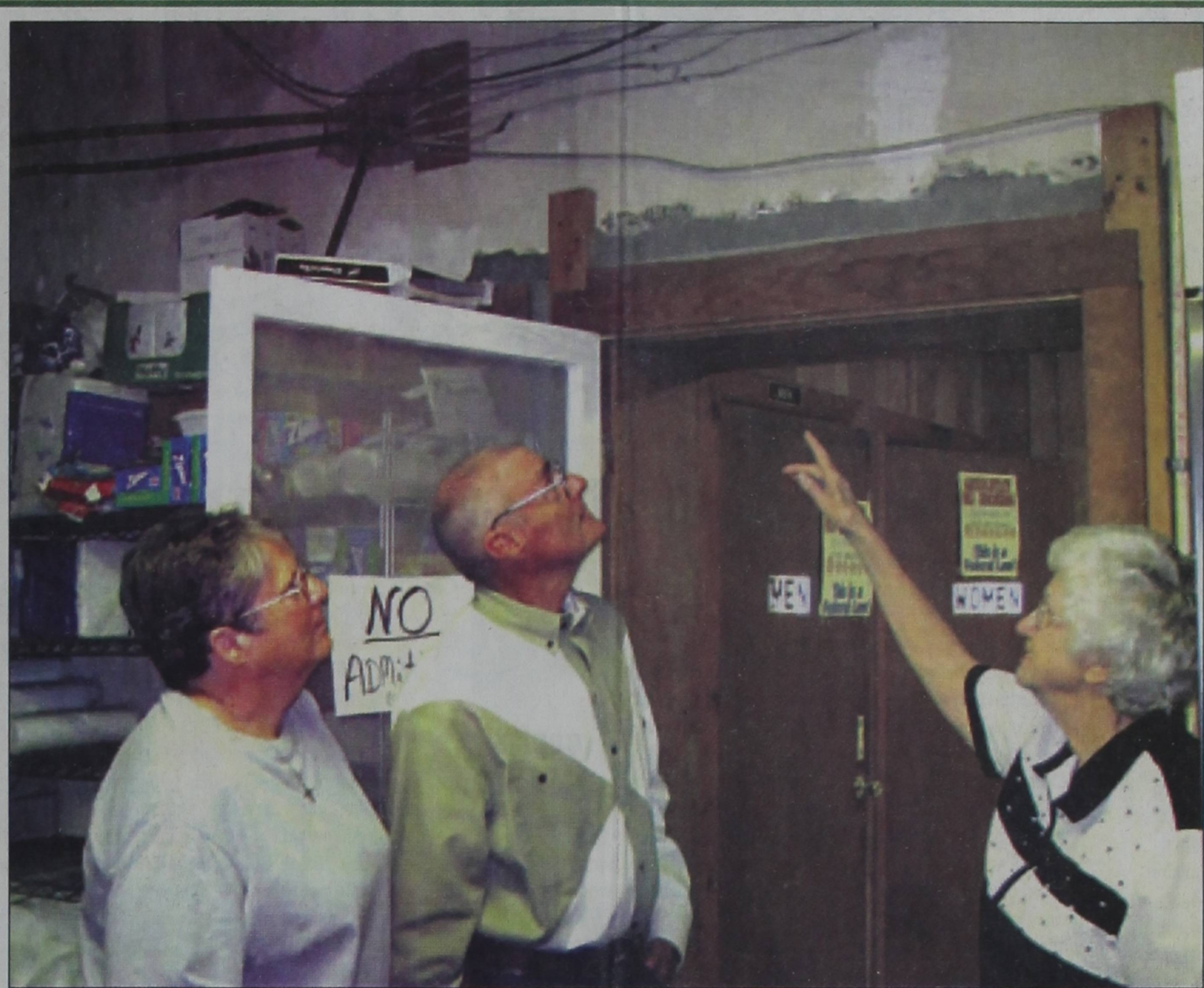
Patsy Spier (right) points out unsafe electrical wiring at the Hedley Senior Citizens Center to Sue and Roger Hagar. Efforts are underway to raise funds for a new senior center in Hedley.
