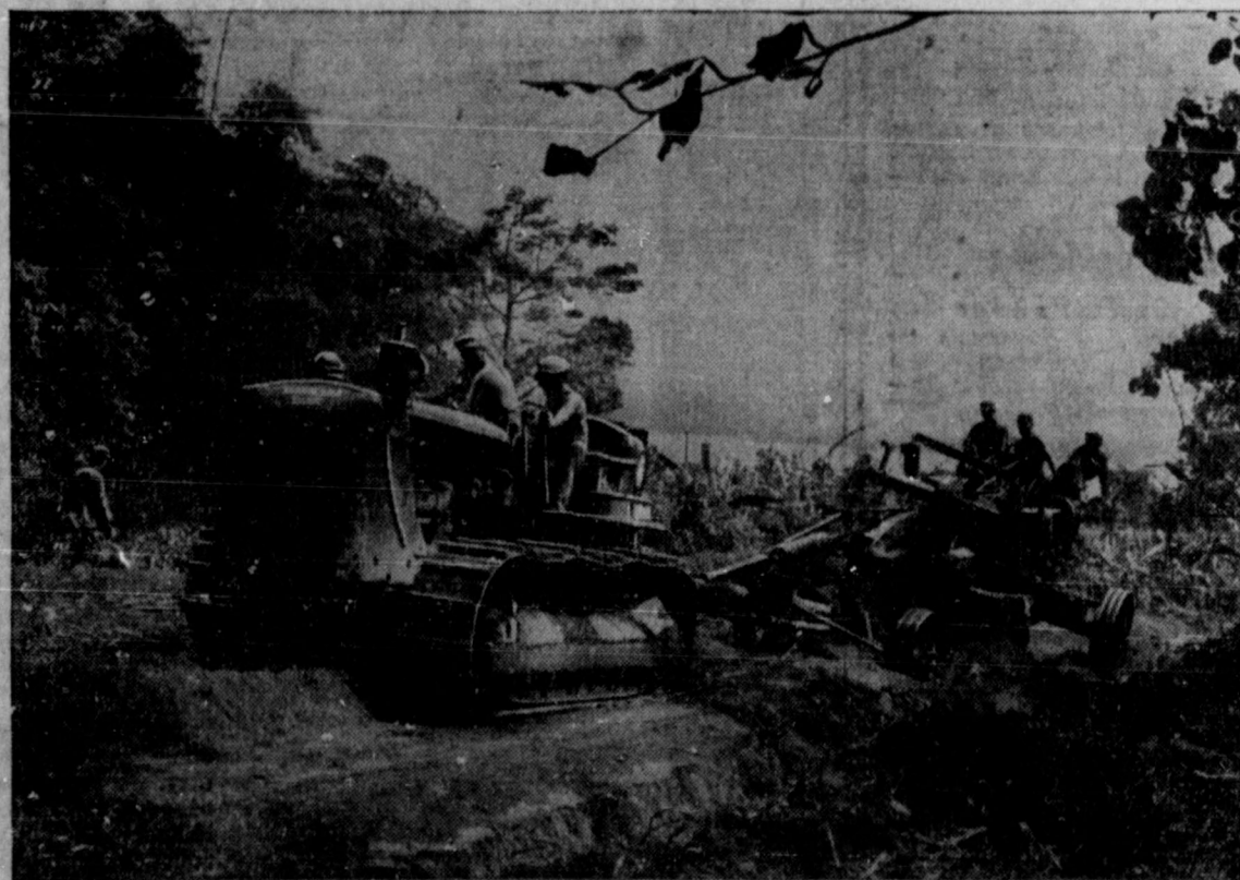
That is the name our engineers call this tractor just as tank men name their tanks and fliers their ships. Starting from scratch these men are driving this road through the jungle in the Sansapor Area of Dutch New Guinea. The tractor is hauling a road grader along a clearing. Your War Bond purchases assure our fighting men of the best of equipment and here you see some of it at work.
