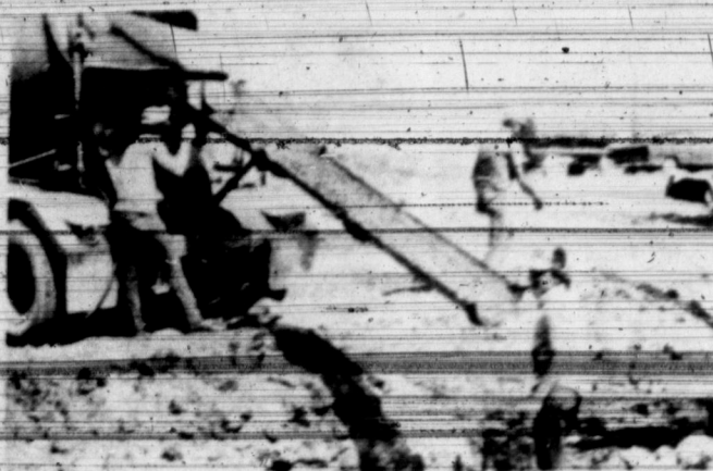
TWO OF FROST'S employes pour quality-controlled concrete into oil-lined steel "treemie" to create a pier.
