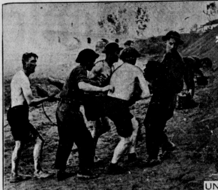
DESPITE THE BOMBS of Nazi planes these British engineers set about repairing a bridge and ford vital to Allied transportation near Medjez-el-Bah. The enemy had dynamited both in retreating and tried, with bombs and shells, to prevent their being repaired again. But the men, stripped to work in the river, stopped only to carry out their casualties, such as the man pictured here who had been hit by a bomb fragment.
