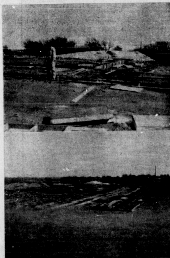
John Jones, local contractor, is on the job and construction is well under way on the new First Baptist Church building here. Second view shows the large area the new church will cover.
