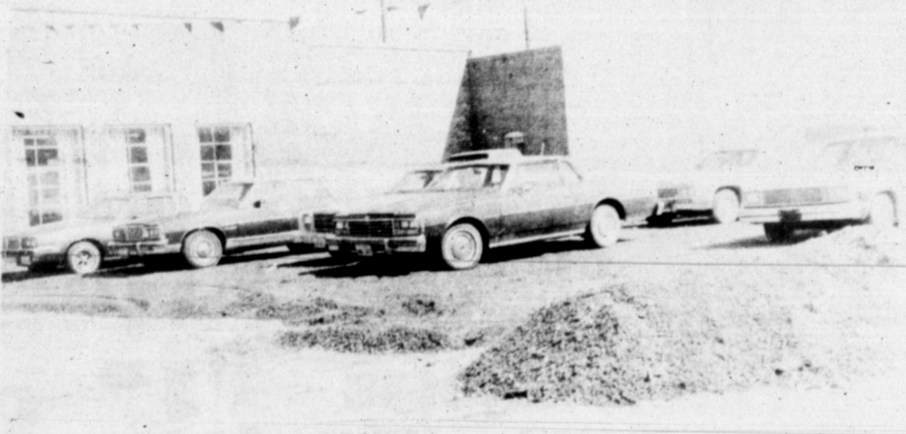
J & J AUTO received a new surface on their parking lot this week.
