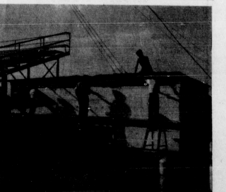
Boys of Scout Troop No. 33 who are working for the Painting Merit Badge are shown as they put a fresh coat of paint on the concession stands at the Rodeo grounds. The buildings were recently acquired by Troop No. 33. Those pictured are David and Richard Leathers, Barry Doan and Jim Bob Thomas. By Saye's
