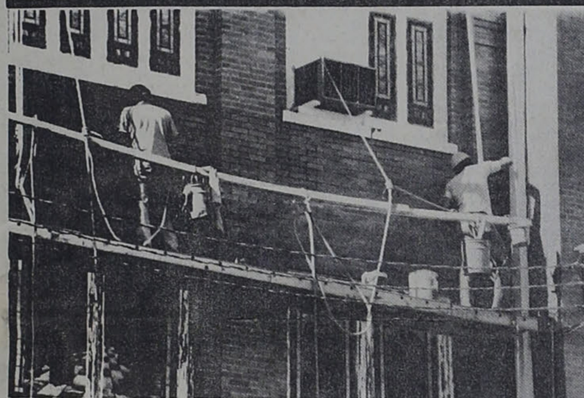
The bricks were cleaned and remortared at the First United Methodist Church. (Photo by Helen Wallace)
