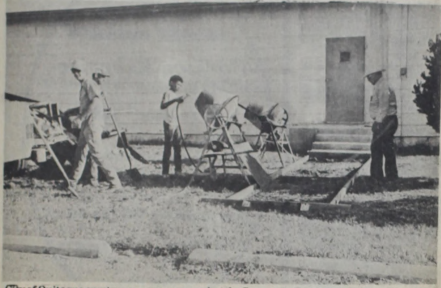
City of Quitaque employees pour a new porch at the Community Center in Quitaque, as they get the building refurbished and ready for Homecoming this weekend. Work was done inside the building, as well as on the outside.
