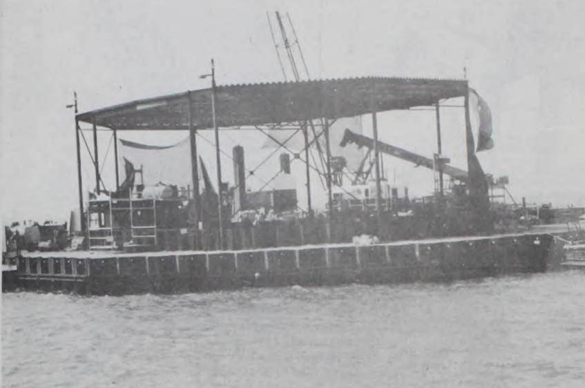
The Cofferdam which is being used for excavation at the site of the LaBelle Ship of La Salle's which was sunk in the Matagorda Bay in 1685.
