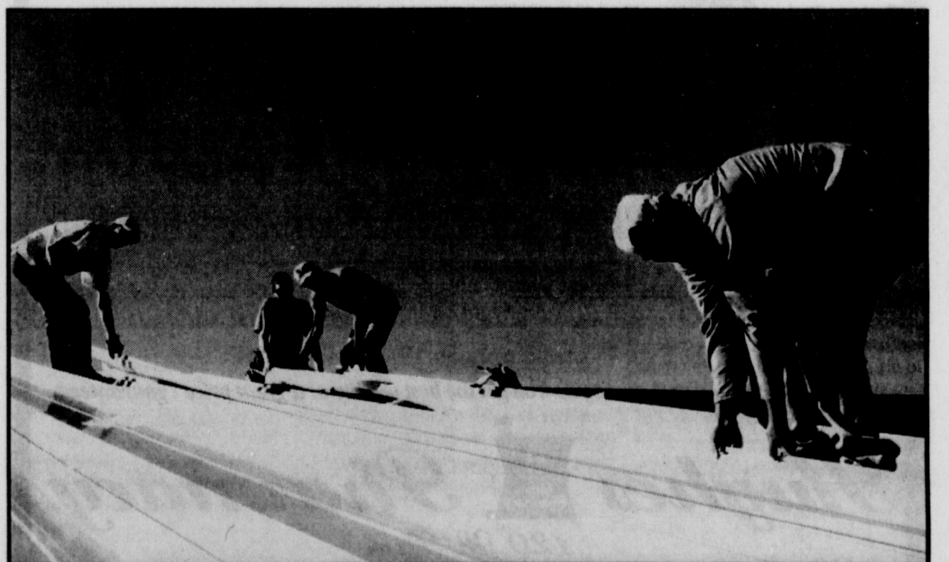
PROGRESS continues on an addition to W.R. Bradford Elementary, with workers finishing the roof of the structure.
