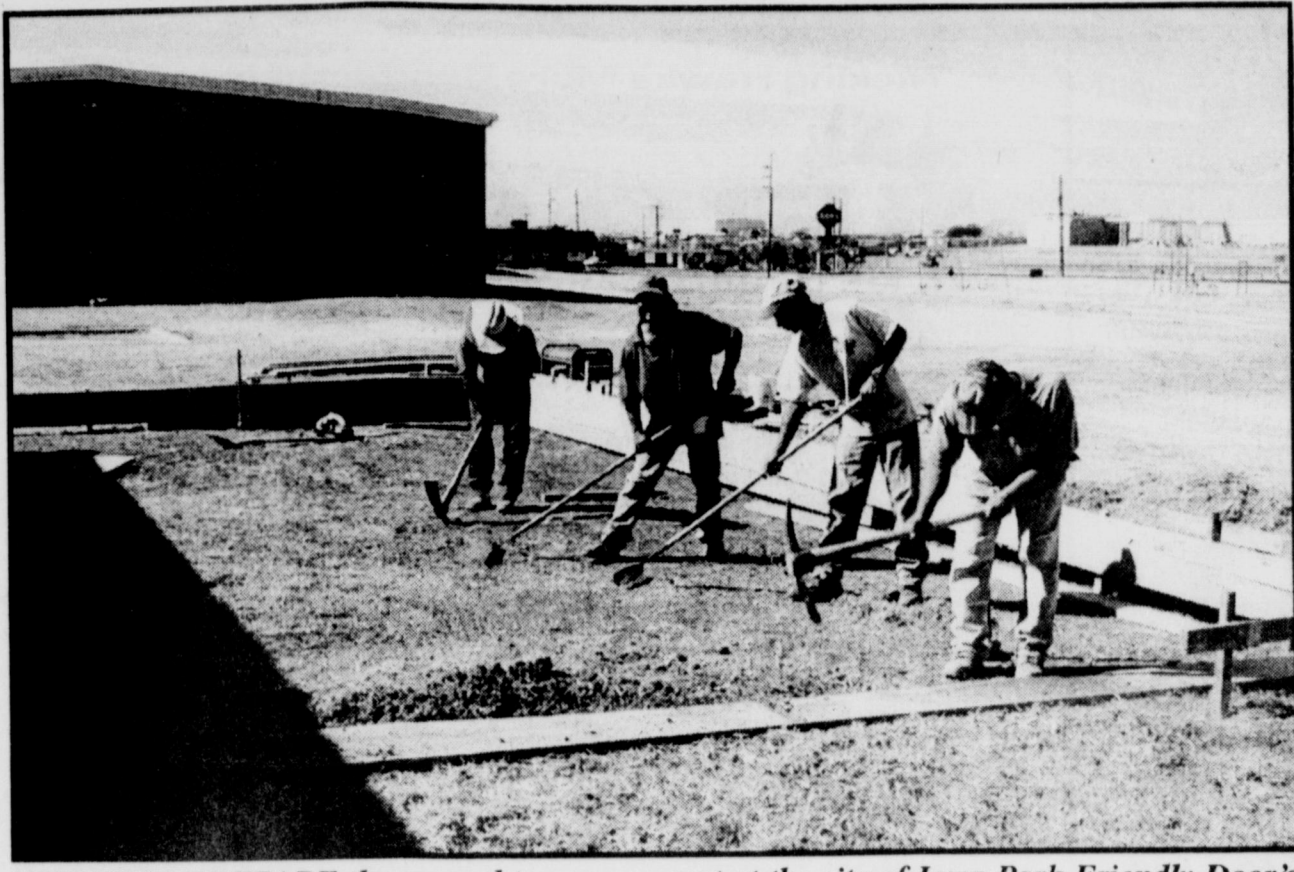
WORKERS PREPARE the ground to pour cement at the site of Iowa Park Friendly Door's kitchen expansion.
