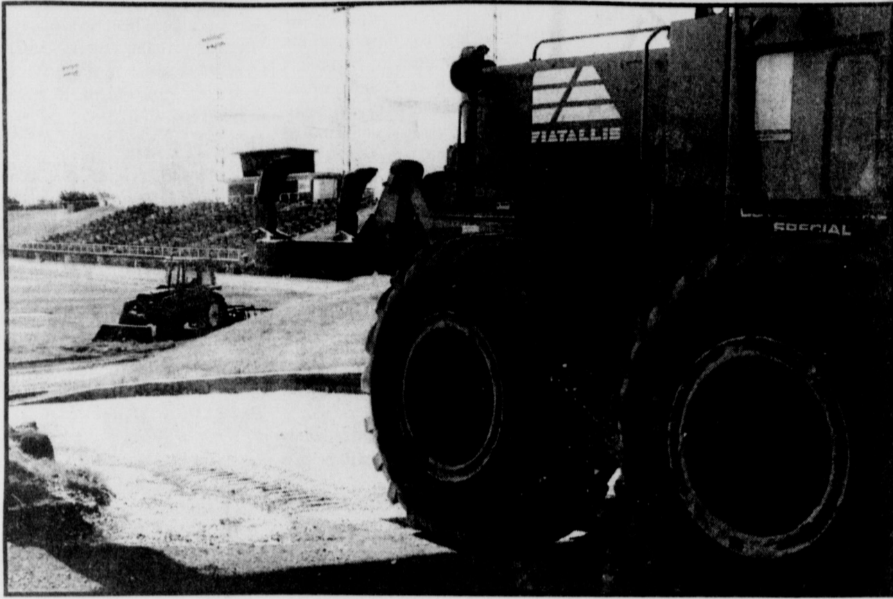
HEAVY EQUIPMENT sat still briefly Tuesday morning, awaiting loads of gravel before final preparations of applying the new surface on the track around Hawk Stadium.
