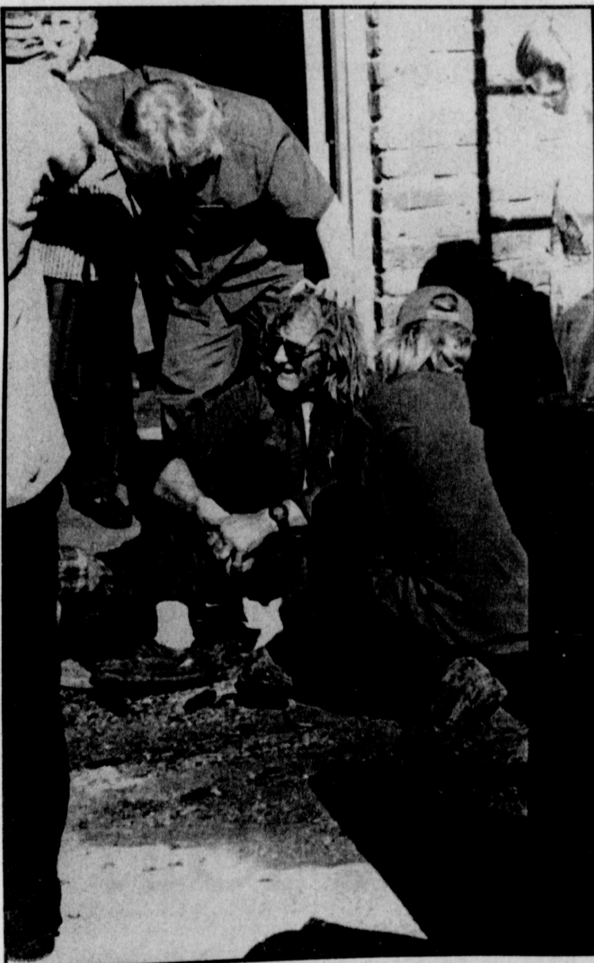
A WORKER sustained only minor injuries when he fell two stories Monday while a roofing firm was working on a building at 117 West Park. His fall was partially blocked by electrical wires. That contact caused the wires to spark, shutting off service to the entire block until repairs could be made. The worker was back on the job Tuesday, however.
