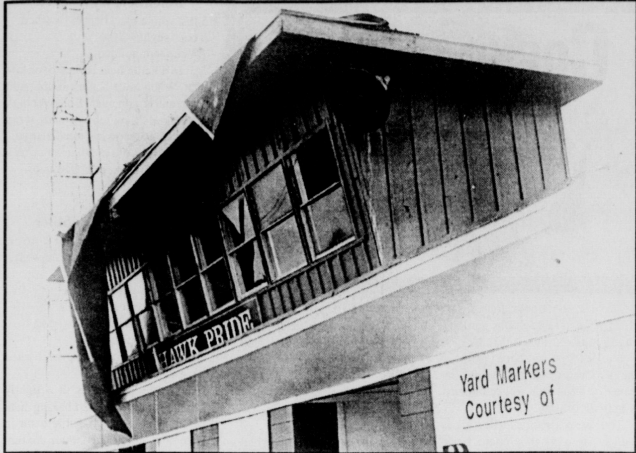
HIGH WINDS that accompanied Sunday afternoon's storm took off much of the roof of the pressbox on the south side of Hawk Stadium. Some damage also was reported on the Junior High campus, and electric service was hampered to most of TU Electric's customers in the east and south part of the city. The storm also deposited .48 of an inch in precipitation.
