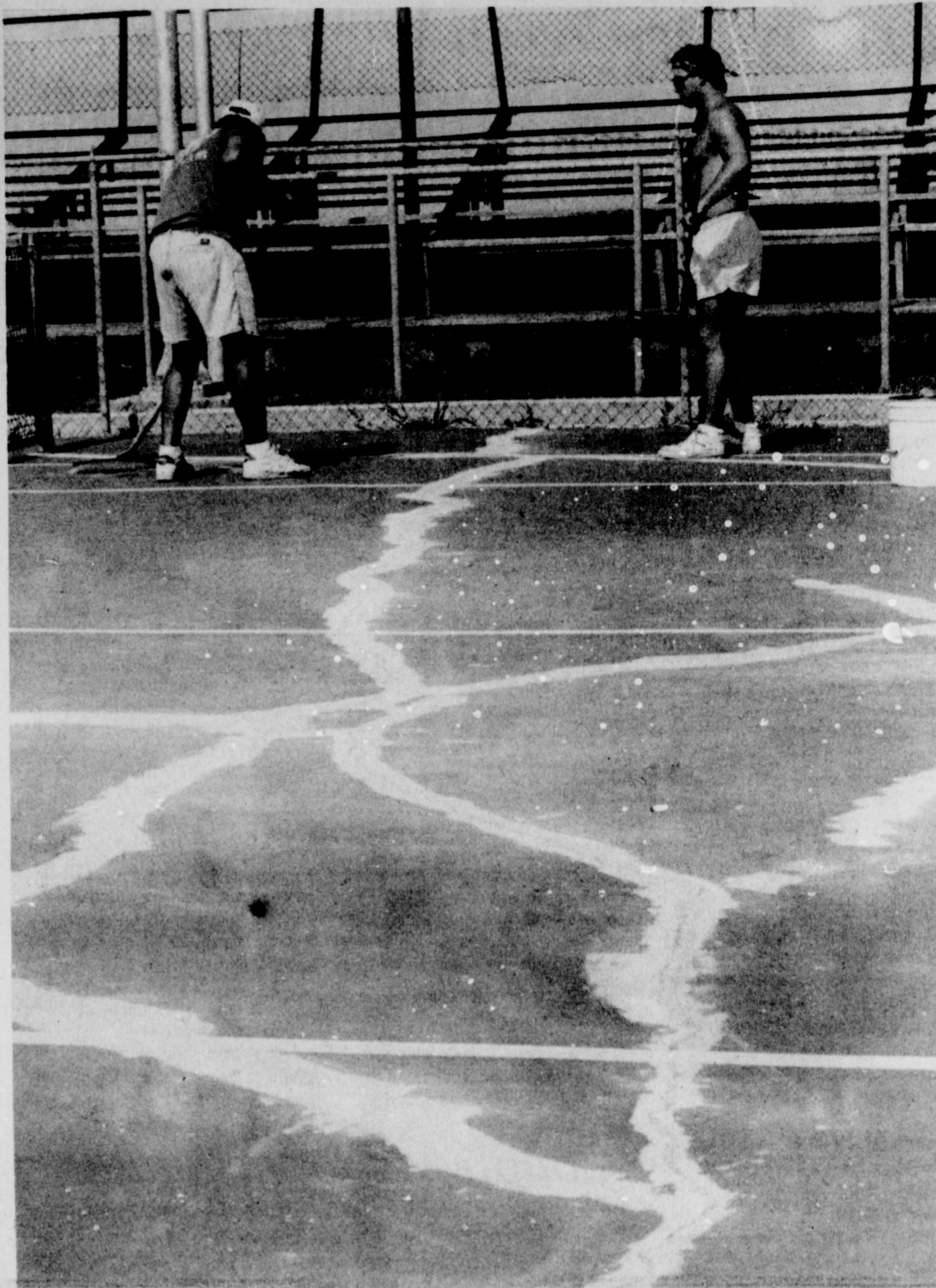
NEARING COMPLETION - Among the numerous preparations for the start of the 1992-93 school year was a project of resurfacing the tennis courts at Iowa Park High School. Coaches Dick Wineinger and John Hoelter have patched cracks, completely repainted the entire concrete surface, and painted new stripes.
