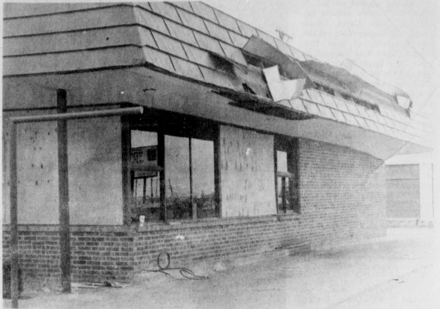
HOLLIDAY DAIRY QUEEN DAMAGE VIEWED FROM OUTSIDE ... following Monday evening storm.
