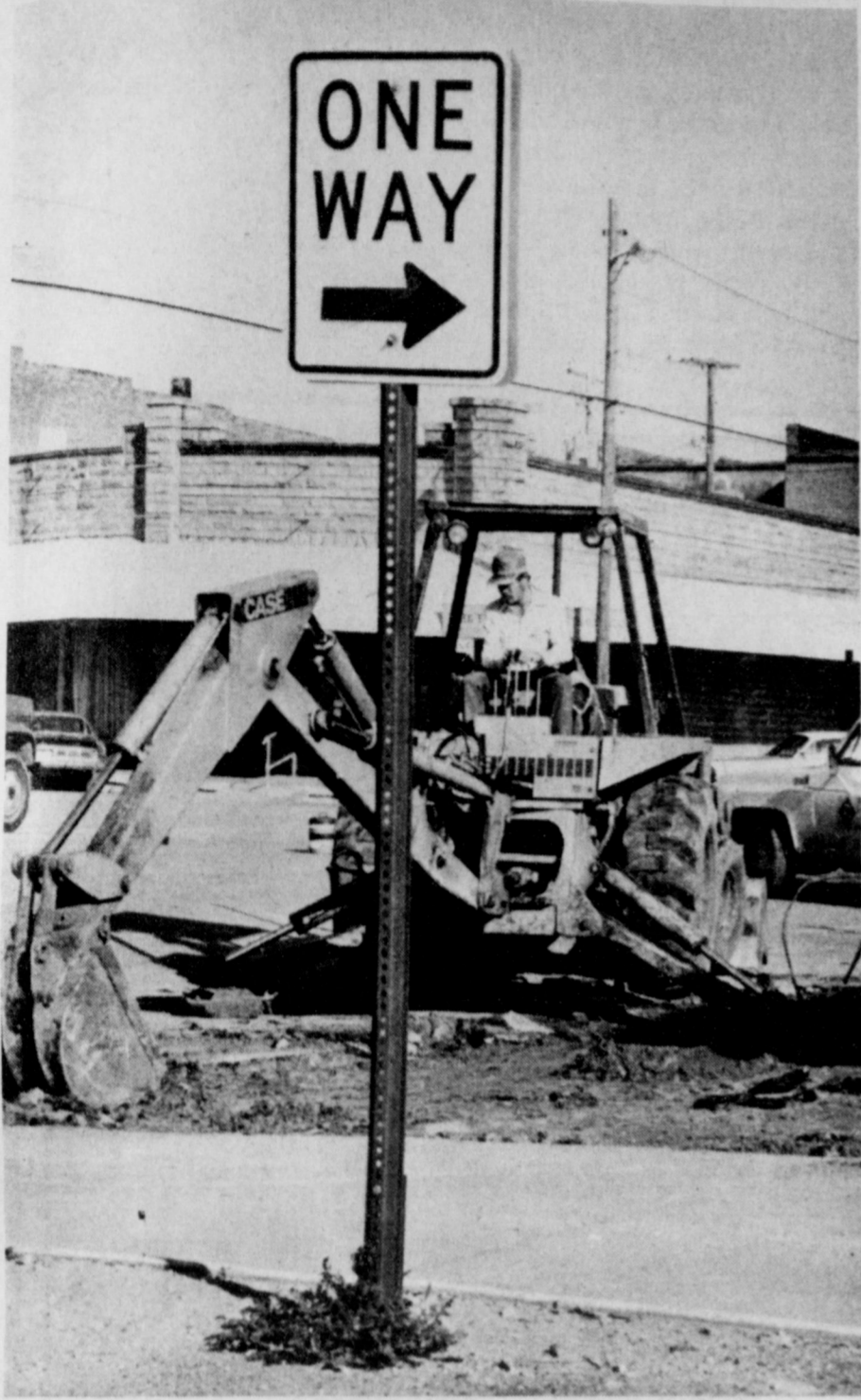
ONE MORE TIME - Traffic into and around city hall was disrupted this week when workers began tearing out the old sidewalk and parking area, to be replaced with concrete. This is the final phase of the city hall renovation project which has been taking place over some eight years.
