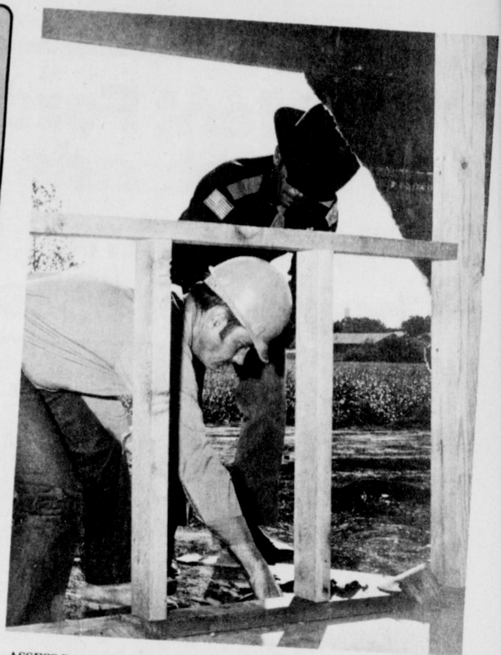
ASSESS DAMAGES--Dexter Parnell, Iowa Park police officer, and Gary Lyles, high school building trades instructor, assess damages to home being built by building trades class on W. Texas. Vandals knocked out large portions of gyp rock siding over the weekend.
