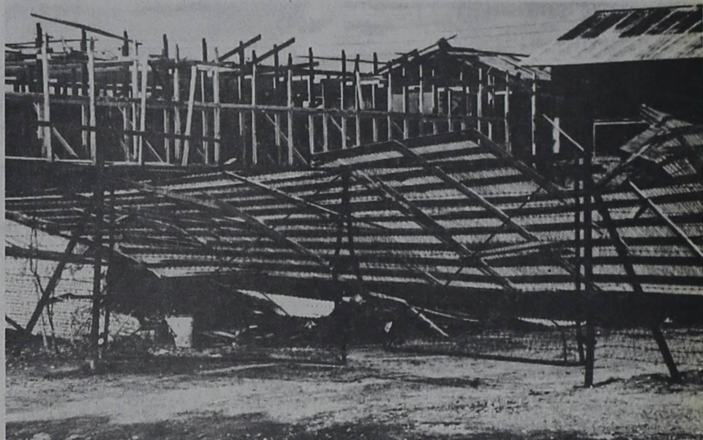
STORM DAMAGE — The old Forrest Lumber Yard on West Eighth street was destroyed in the late Tuesday storm which struck Post about 9:30 p.m.
